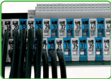
Terminal strips placed behind each other save space – staggering them by half the pin spacing simplifies subsequent wiring of the first row.
