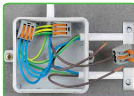
Wiring of flexible conductors in a junction box.
