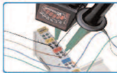
Signal tracing with wired conductors
