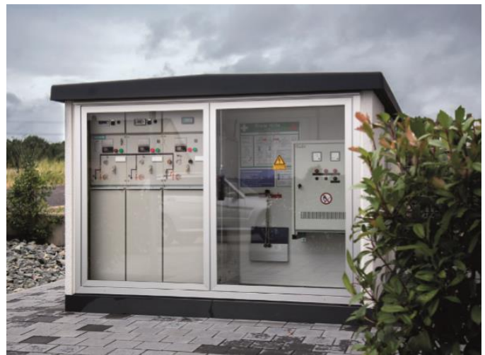
The path to making a smart grid: The intelligent local network station from the engineering firm Pfeffer enables measuring, controlling, regulating and remote control using components from WAGO
